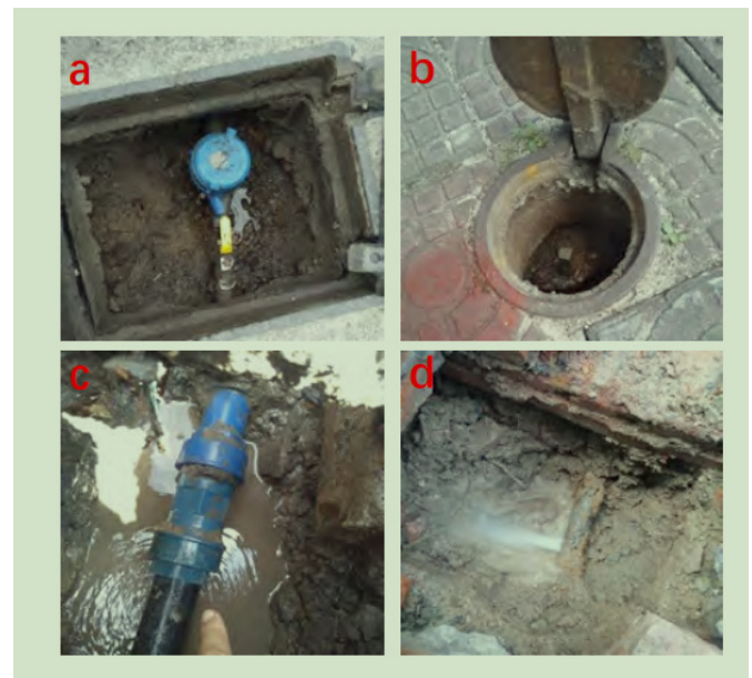
Figure 9: On-site photos of satellite detection leaks
